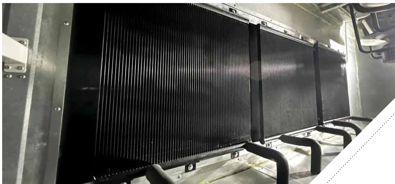
Installed a heat recovery system to reduce SETSCO's energy consumption.
